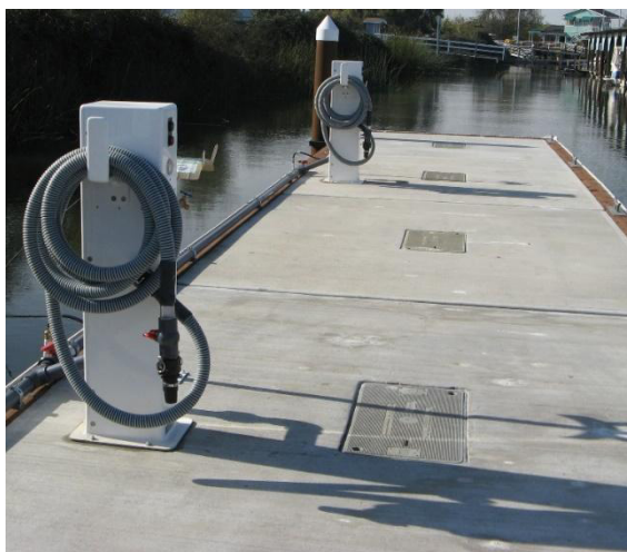
Image 3: Sewage pump in the marina (nautical port). Copengahen, Danska
