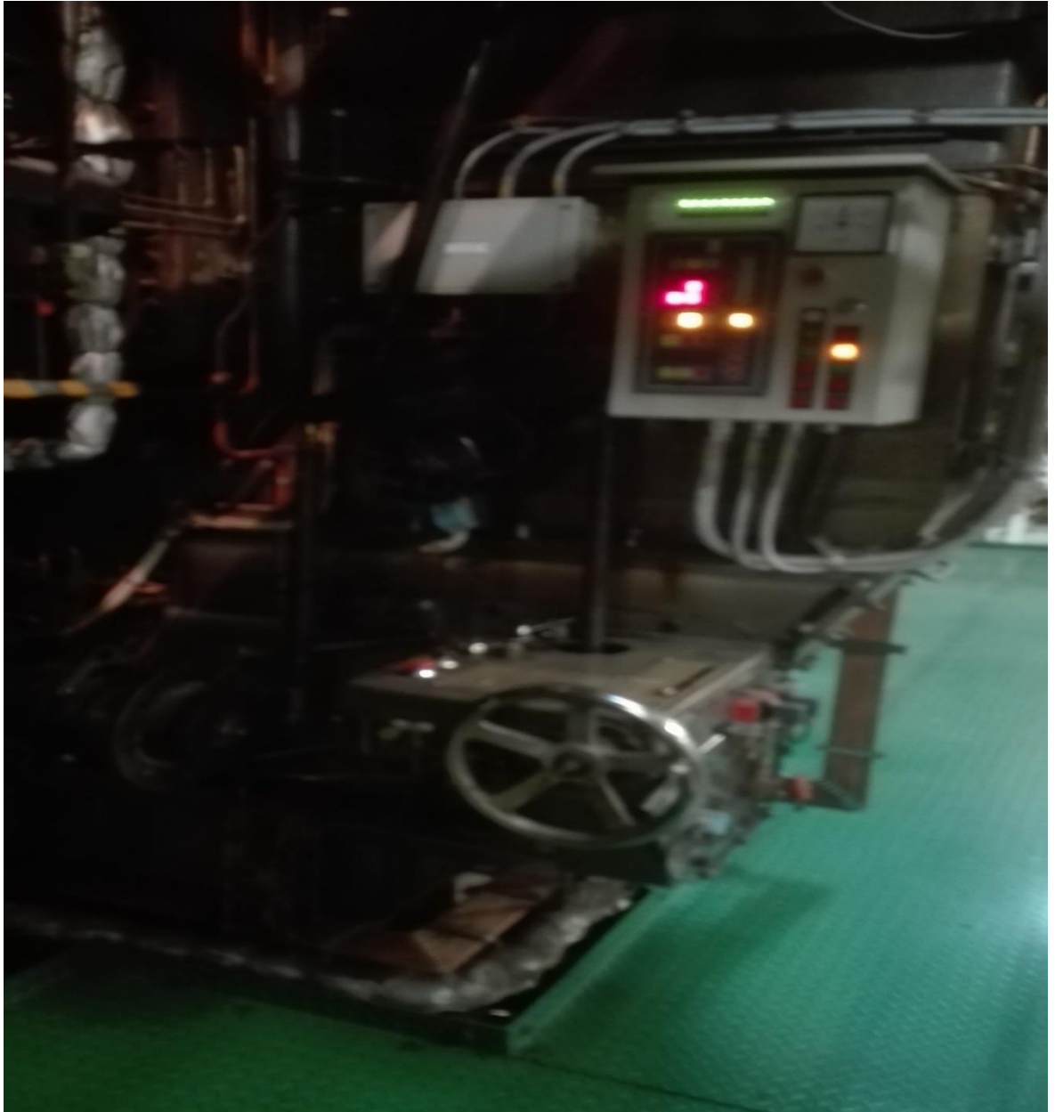
Figure 18 Engine local control console vessel MV NORDAUTUMN
