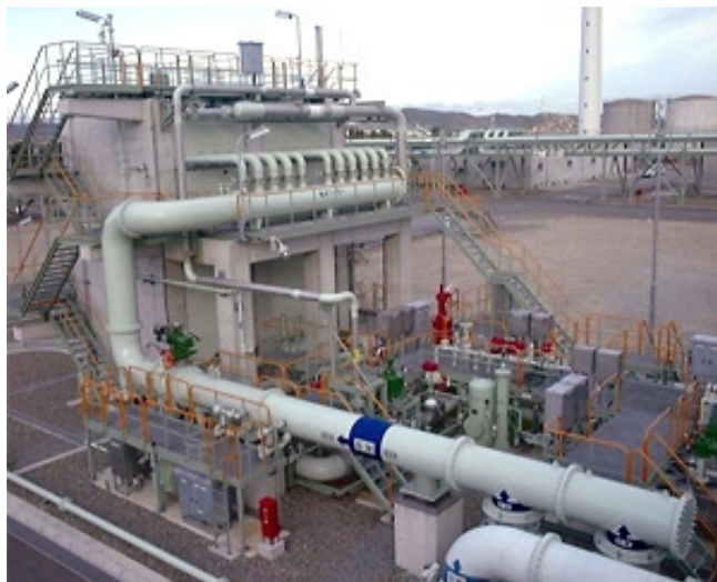
First commercial SUPERORV (Osaka Gas Himeji terminal)
