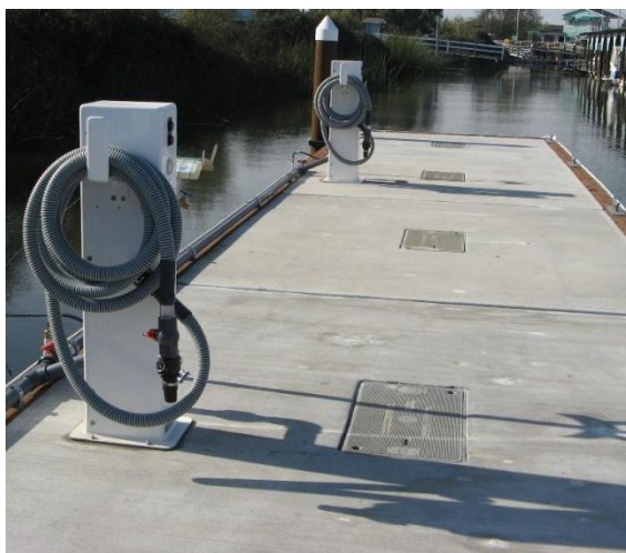
Image 3: Sewage pump in the marina (nautical port). Copengahen, Danska
